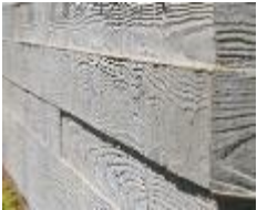
adze textured concrete
